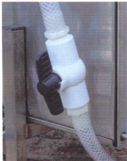
Figure 24: Background shutoff valve in the "OPEN" position.
