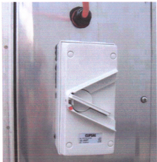
Figure 23: Blower shutoff switch in the "ON" position.
