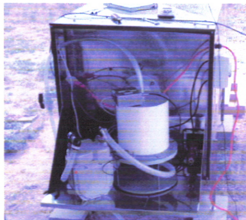
Figure 8: Electronics enclosure open.
