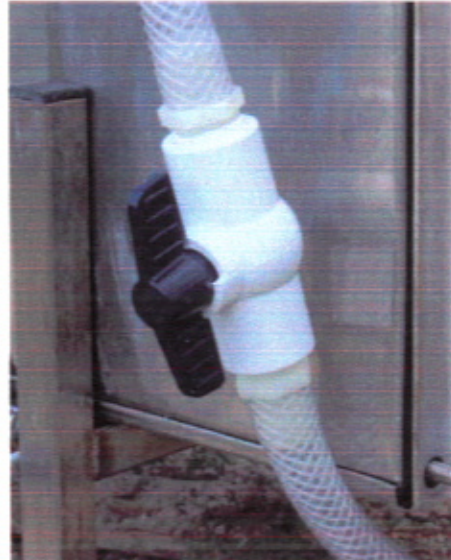
Figure 24: Background shutoff valve in the "OPEN" position.
