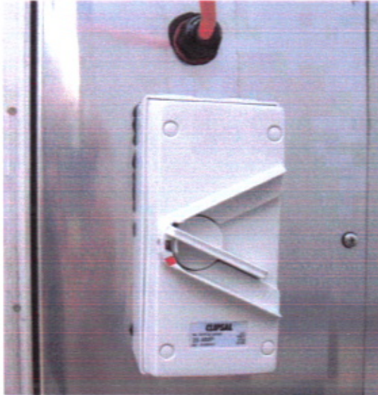
Figure 23: Blower shutoff switch in the "ON" position.
