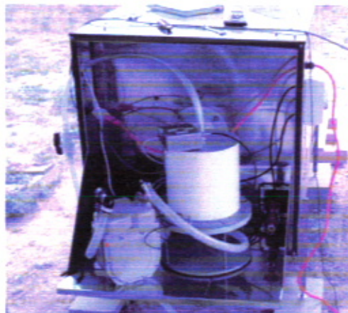
Figure 8: Electronics enclosure open.
