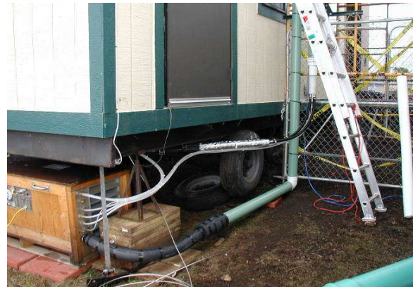
Figure 2-4: Pumpbox at Trinidad Head. Shelter from rain is provided by installing the pumpbox under the elevated instrument trailer at this site.
