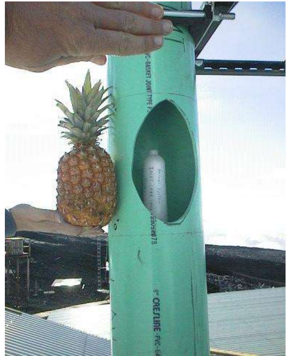
Figure 3-5: Close up view of stack access port at Mauna Loa, with HEPA capsule filter installed on aerosol inlet.
