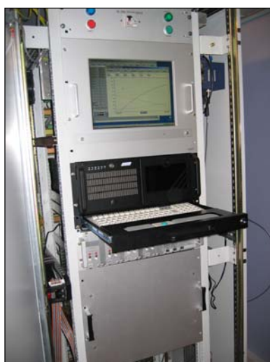
Figure 1: View of the analysis compartment. Industrial standards have been chosen for high robustness, and easy maintainability.
