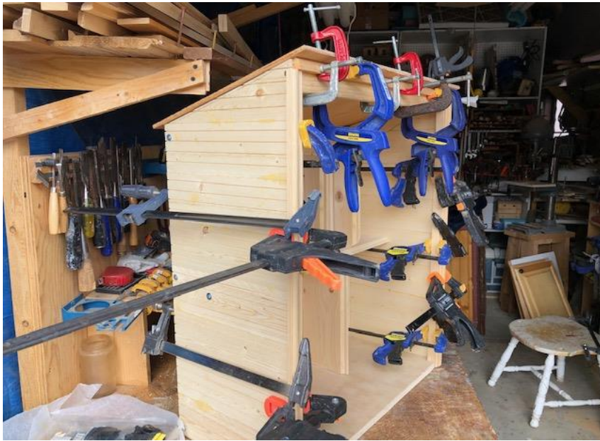
Figure 23. (Upper) Ugandan LFL under construction held together with glue instead of heavier screws.
