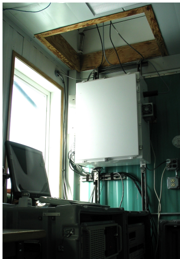
Figure 2.7. The SUV-150B spectroradiometer installation at Summit Greenland. The monochromator enclosure (white box) is mounted on the wall. The collector is installed into a roof hatch above the instrument. System control computer and additional electronic equipment are installed in separate racks in the foreground.
