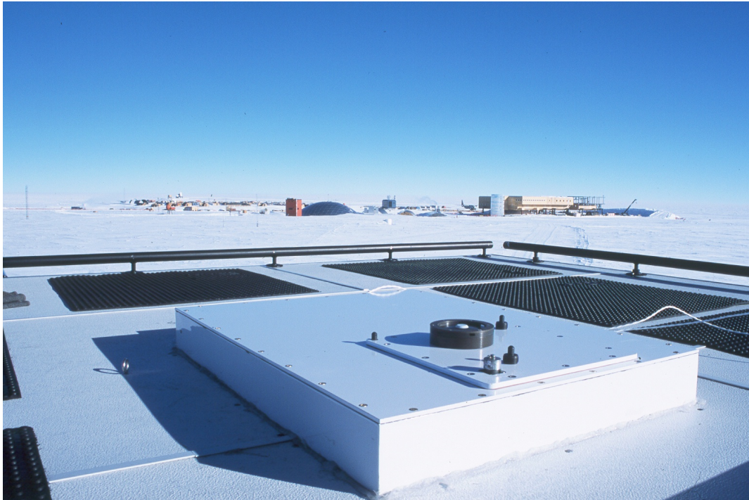
Figure 3.3.1. Top of the SUV-100 spectroradiometer installed into the roof the Atmospheric Research Observatory (ARO). In the background, the dome of the Amundsen-Scott South Pole Station and the building of the new station, which is currently under construction, can be seen. The pictures was taken in January 2002.
