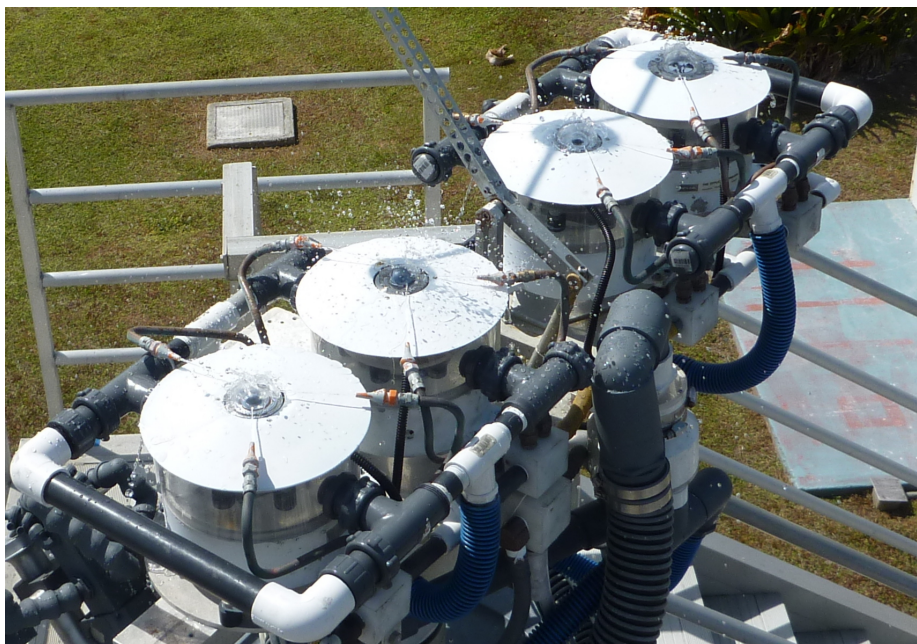
Figure 1. A view of the sensor wash cycle in operation at the Kwajalein BSRN site. The sensor domes are sprayed with water obtained from a fresh water line inside the building on which the tracker is mounted. Each cycle lasts about 15 seconds and is turned on and off via software in the data logger program. The sensors are ventilated using conditioned air pumped continuously by regenerative blowers located inside the building. Two blowers are used to add redundancy.
