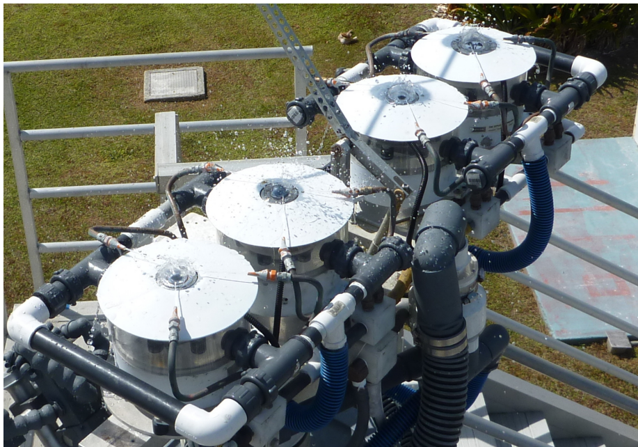
Figure 1. A view of the sensor wash cycle in operation at the Kwajalein BSRN site. The sensor domes are sprayed with water obtained from a fresh water line inside the building on which the tracker is mounted. Each cycle lasts about 15 seconds and is turned on and off via software in the data logger program. The sensors are ventilated using conditioned air pumped continuously by regenerative blowers located inside the building. Two blowers are used to add redundancy.
